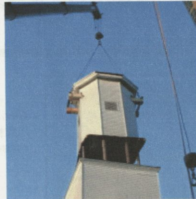
Lift-off: A Pownal Center Community Church bell tower was removed from its base on Sept. 27.
